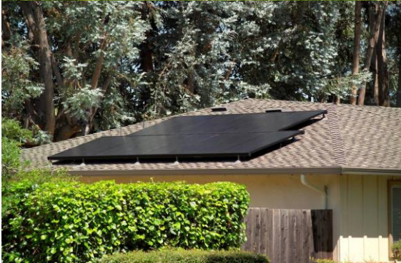
(Noncompliant street side roofs with exposed and metallic mounting hardware and lack of symmetry in application of equipment.)
